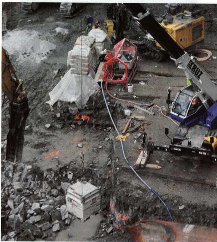
Workers lower a Transcube fuel transportation tank into the hole at the World Trade Center Memorial site. Contractors began using Transcube tanks after a modified tank spilled fuel while being moved.
