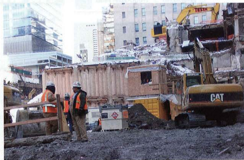
TOP: The Transcube tanks provide secondary containment with an outer wall structure completely enclosing the inner tank. ABOVE: Several companies are performing excavation and foundation work at the WTC Memorial site. Contractors are using the Transcube tanks to bring diesel down from grade level to fuel their machines.
